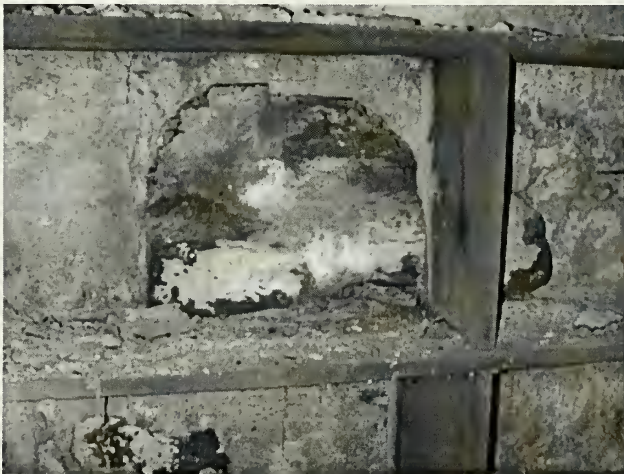
Figure 11 Stone Jutting from the Interior Masonry Wall in the Basement of the Center Section of the Main House, 2002
